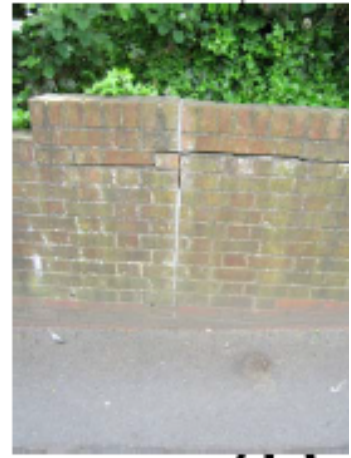
Horizontal crack for repair.
