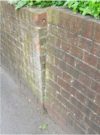
Horizontal displacement at movement joint.
